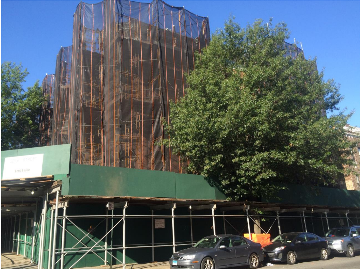
Corner of Eighth Avenue and Fifth Street. Scaffolding and sidewalk bridge has been installed.
